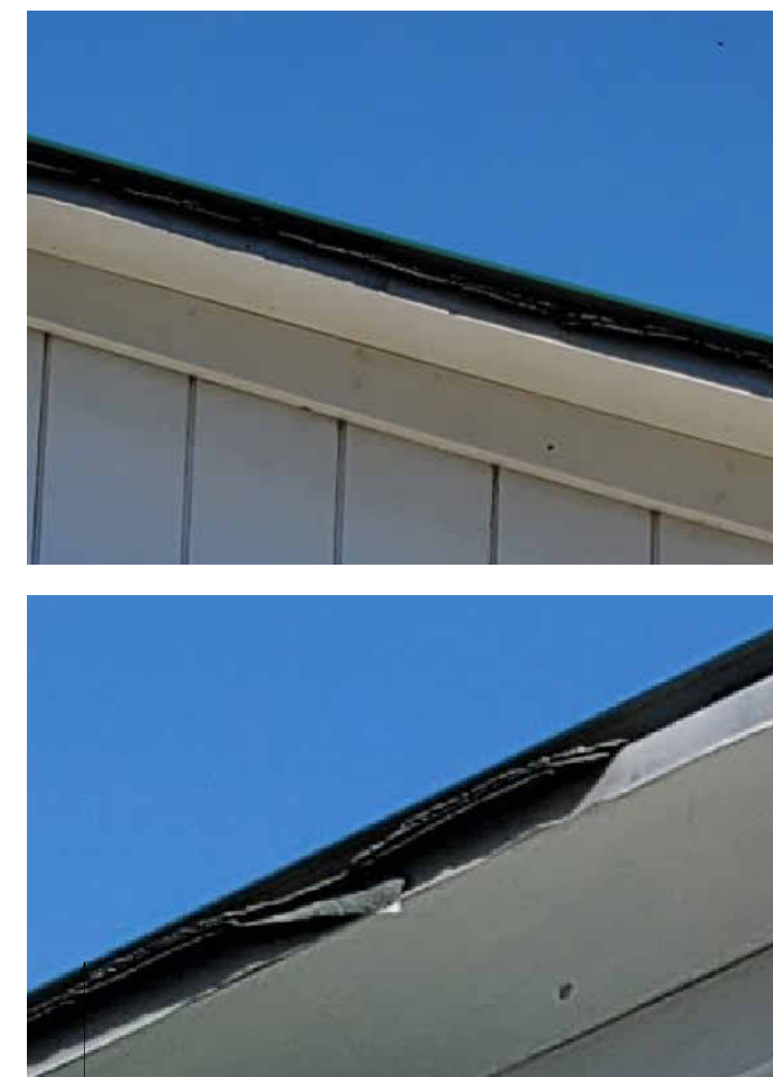
EVIDENCE OF ASPHALT SHINGLES. REMOVE STANDING SEAM METAL ROOFING AND ASPHALT SHINGLES DOWN TO SHEATHING. INSTALL ICE AND WATERSHIELD MEMBRANE AND REPLACE WITH NEW STANDING SEAM METAL ROOFING
