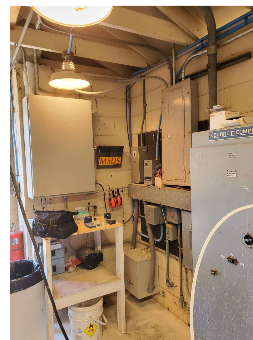
PHOTO 12: LOOKING SOUTHEAST TOWARD ELECTRICAL PANEL
