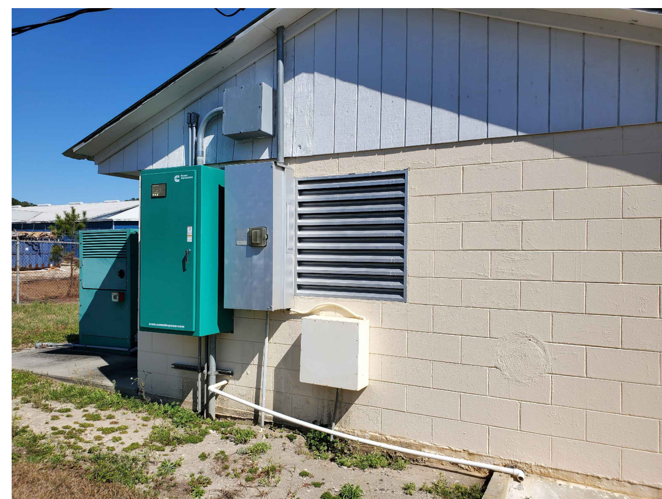
PHOTO 10: LOOKING EAST TOWARD CONTROL PANEL
