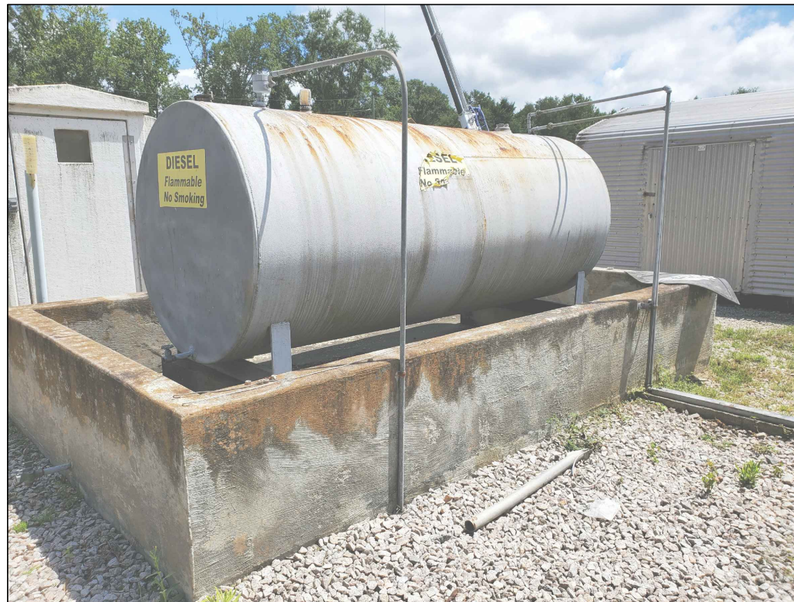
EXISTING 1000 GALLON FUEL TANK AND CONTAINMENT (SHOWN INSTALLED AT FORMER LOCATION AT JIMMY MIXSON WRF)
