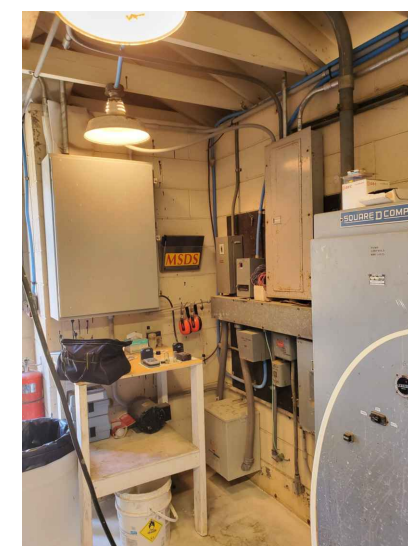
PHOTO 12: LOOKING SOUTHEAST TOWARD ELECTRICAL PANEL
