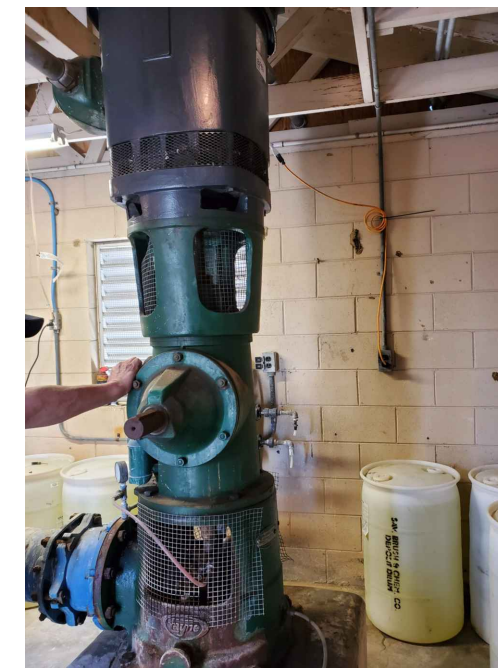
PHOTO 6: LOOKING WEST TOWARD WELL PUMP
