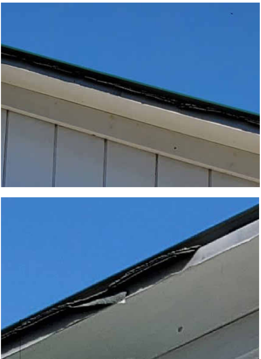
EVIDENCE OF ASPHALT SHINGLES. REMOVE STANDING SEAM METAL ROOFING AND ASPHALT SHINGLES DOWN TO SHEATHING. INSTALL ICE AND WATERSHIELD MEMBRANE AND REPLACE WITH NEW STANDING SEAM METAL ROOFING
