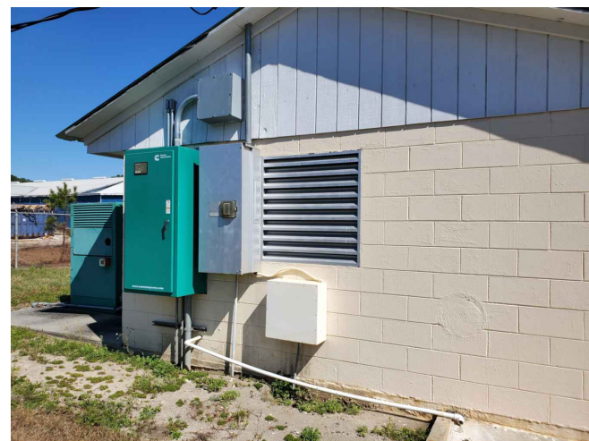
PHOTO 10: LOOKING EAST TOWARD CONTROL PANEL
