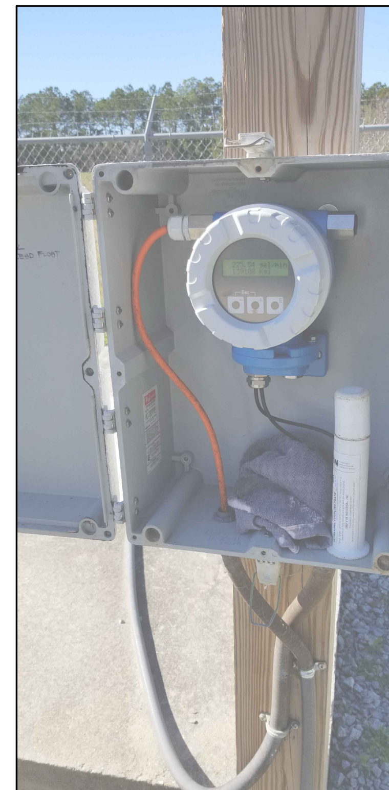
PHOTO-7 LOOKING WEST AT FLOW METER TRANSMITTER BOX ADJACENT TO VALVE VAULT
