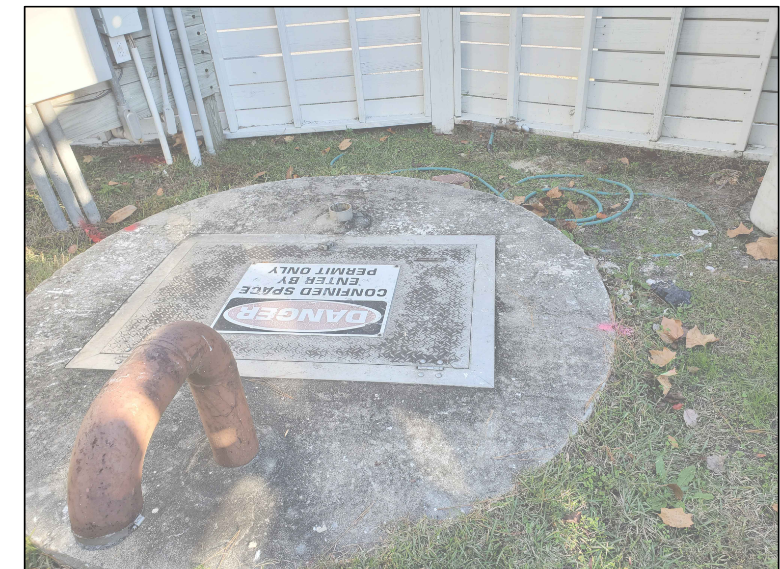
PHOTO-6 LOOKING EAST AT WET WELL
