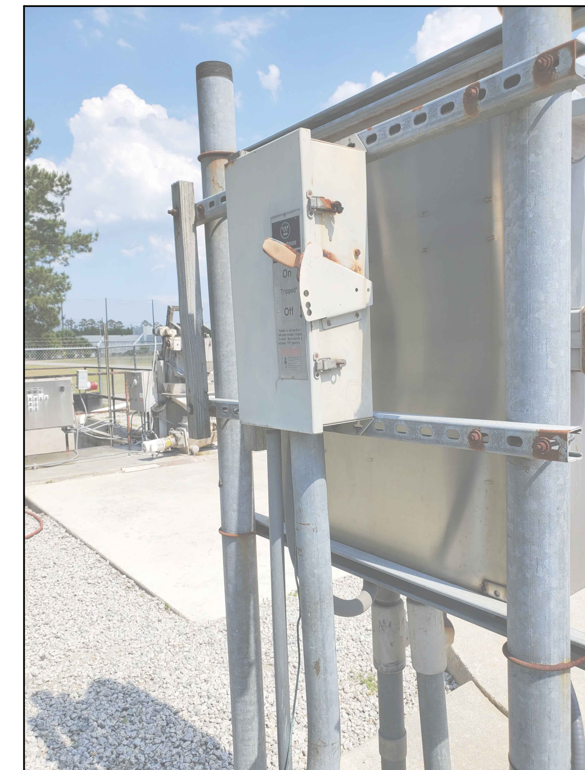
PHOTO-9 LOOKING SOUTHEAST AT BACK OF PANEL RACK
