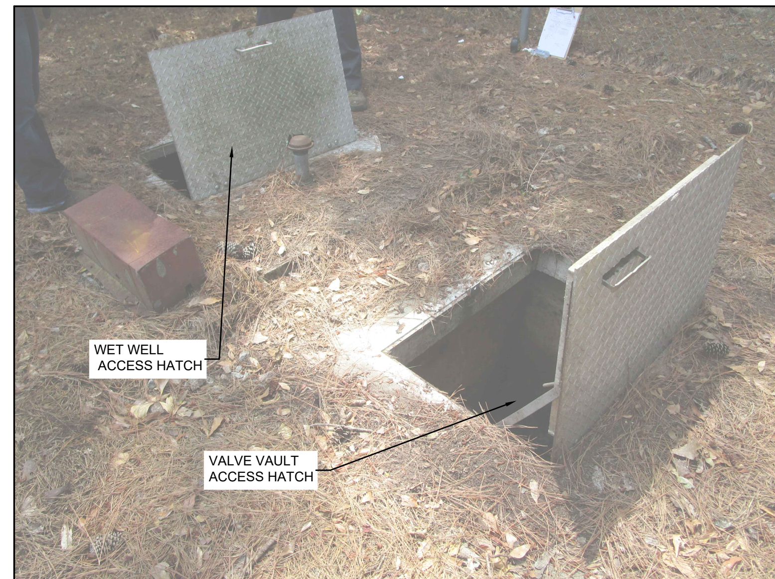
PHOTO-7 LOOKING SOUTH AT WET WELL AND VALVE VAULT
