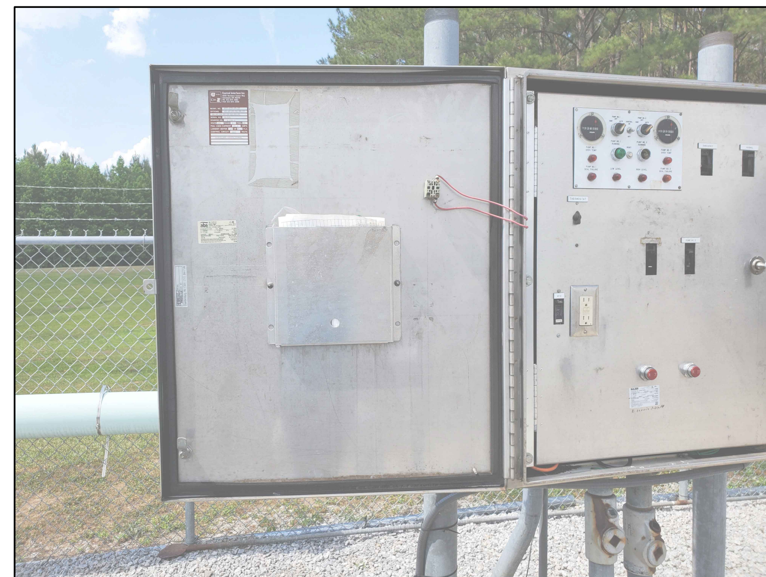
PHOTO-8 LOOKING NORTH AT PUMP STATION CONTROL PANEL
