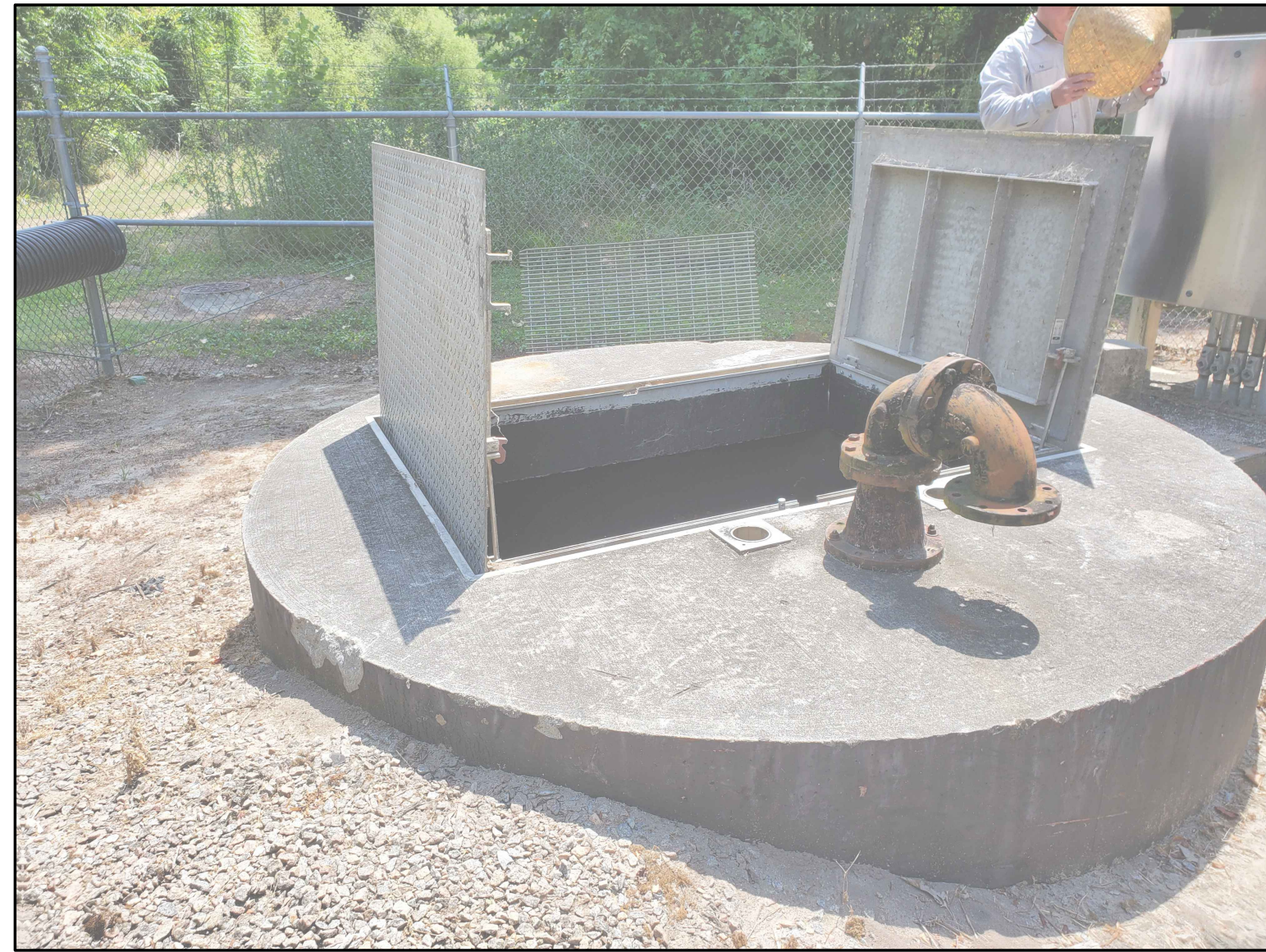
PHOTO-5 LOOKING SOUTHEAST AT WET WELL
